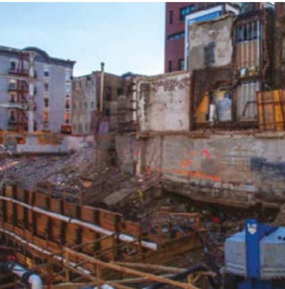
FIGURE 1 – PROJECT SITE AT 150 CHARLES STREET AFTER HURRICANE SANDY (OCTOBER 2012)
